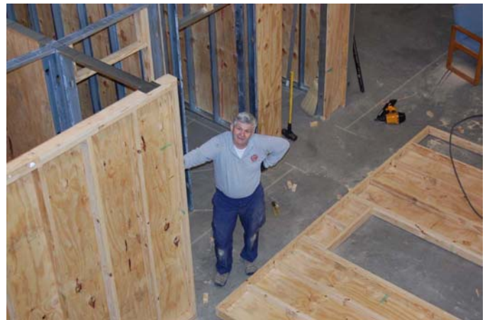
Bob Tokarchic framing the walls that are part of the new practical training area.
