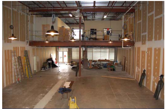
Pre construction phase, after the area had been cleared. The “Un-built” area has been used for various purposes over the years and had taken on the appearance of a cluttered un-finished basement.
