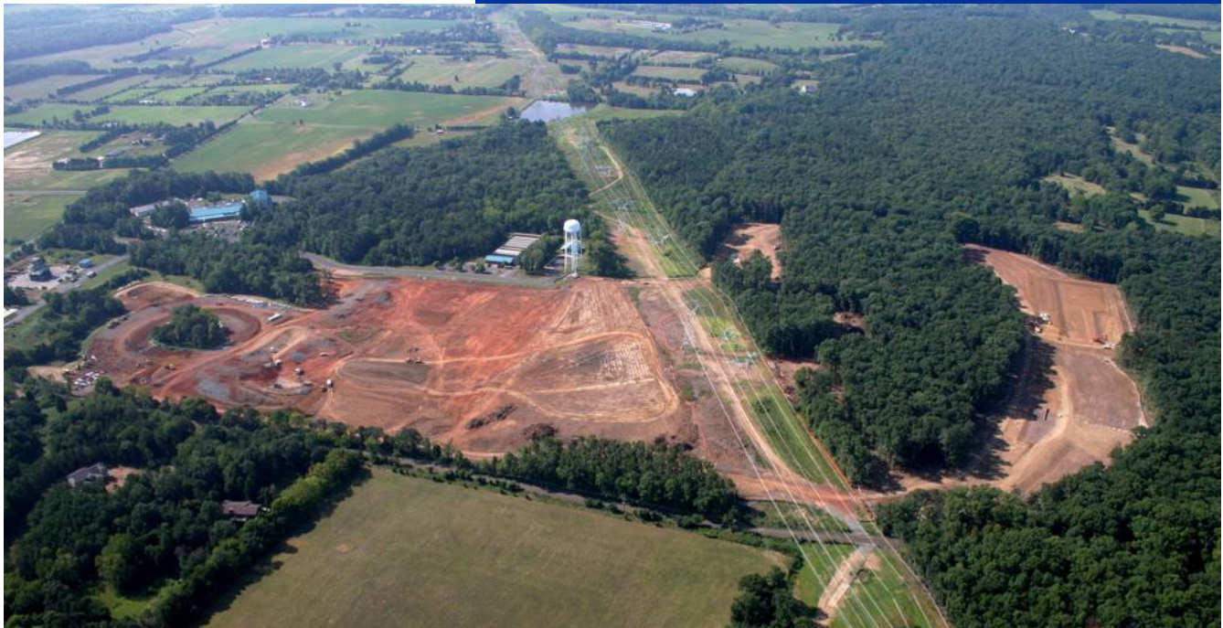
Site work for the new track. The cleared area outlines the track configuration.
